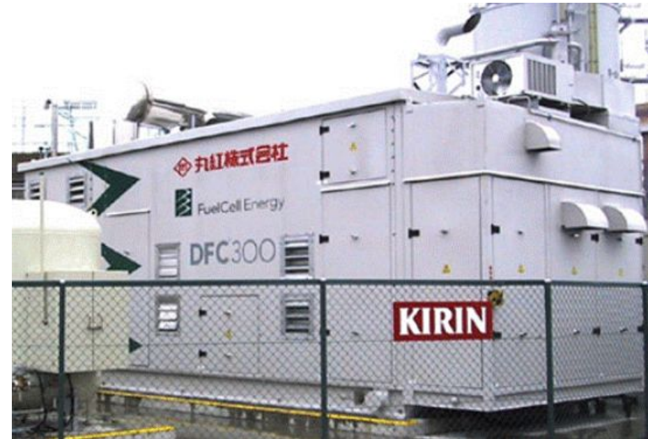
250kW Carbonate CHP Powerplant deployed at Kirin Brewery, Japan, in 2003
