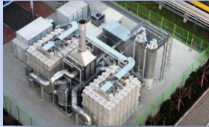
2.8 MW net power 47% electrical efficiency up to 90% total efficiency
