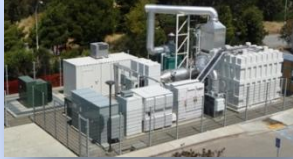
1.4 MW net power 47% electrical efficiency up to 90% total efficiency
